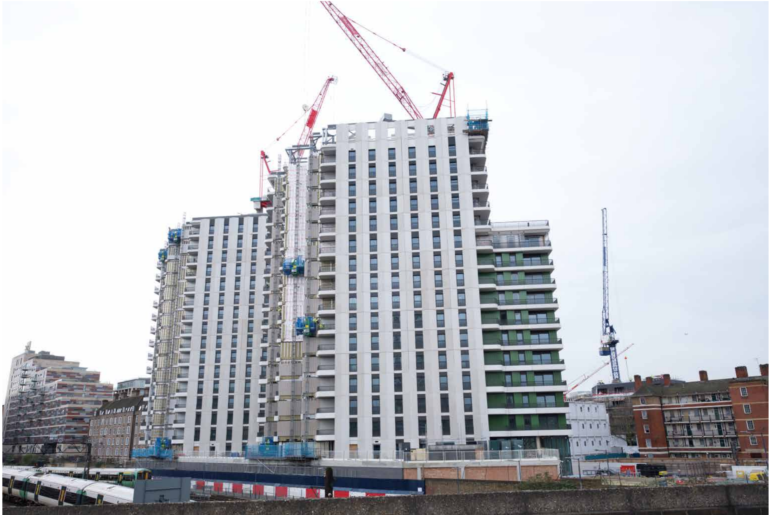
Above: photograph from phase 1 under construction on site, showing side elevations of Tall Buildings
